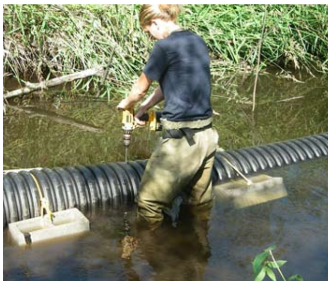
Drilling holes in a flex pipe allows air to escape so it sinks.
